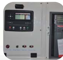
Control Panel & MCB
